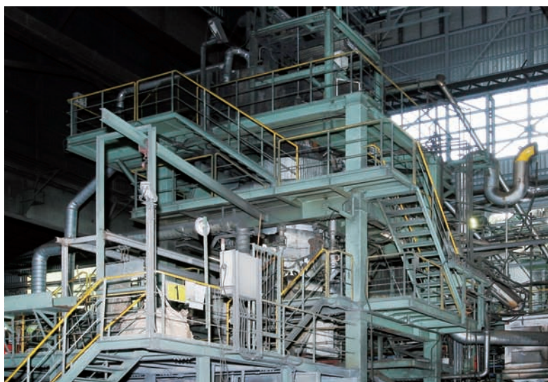
Pyro-metallurgical process within the HMC project (copper recovery furnace)
