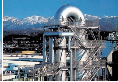
Gasification melting furnace (Nikko Mikkaichi Recycle Co., Ltd.) [Toyama Prefecture]
