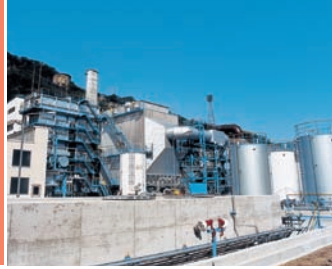
Clean Z furnace (Nikko Environmental Services Co., Ltd.) [Ibaraki Prefecture]
